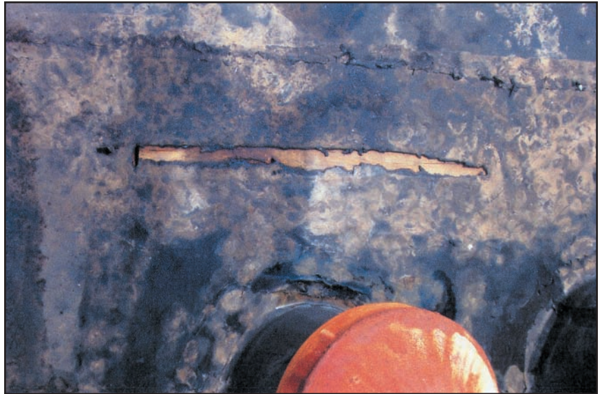
Figure 6: A 15-year-old EPDM with a severe tear caused by shrinkage over time.
