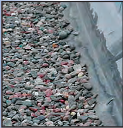
Before - Tenting of EPDM membrane at perimeter wall due to loss of attachment of membrane to base tie-in.
