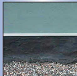
After - Repaired open joint in flashing by using the three-course flashing repair method.
