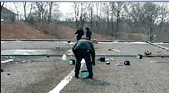
Repair of split membrane by using a three course flashing repair method, consisting of a base layer of plastic cement, a layer of asphalt coated fabric and a top layer of plastic cement.
