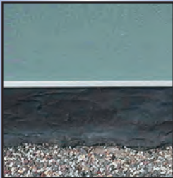
After- Installation of new Reinforced Perimeter Flashing Strip with butyl tape attached and EPDM flashing. New EPDM flashings are seamed to the underside of the existing EPDM field membrane.
